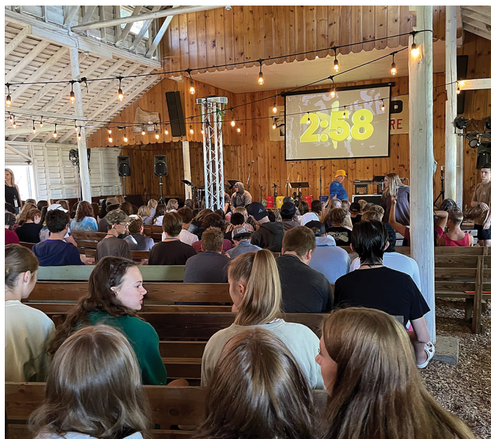
Tabernacle at Camp Sanders needs major renovations. Photo courtesy of the camp
